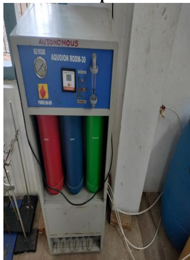
Ion exchange Distilled water plant
